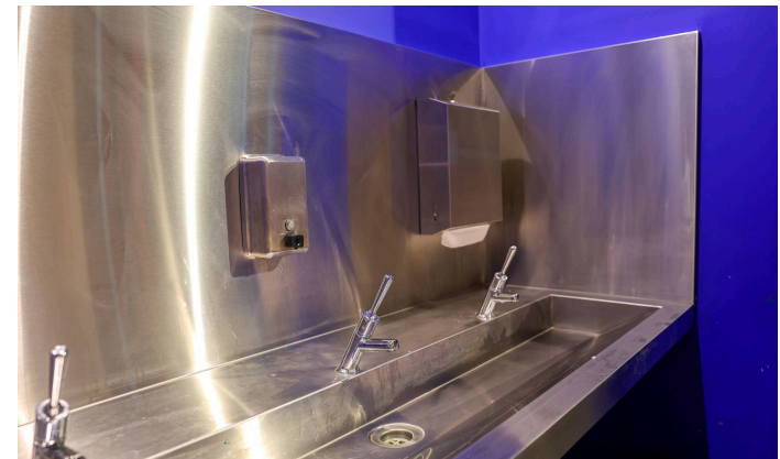
Stainless steel sink trough with three push taps, soap and paper towel dispensers.
