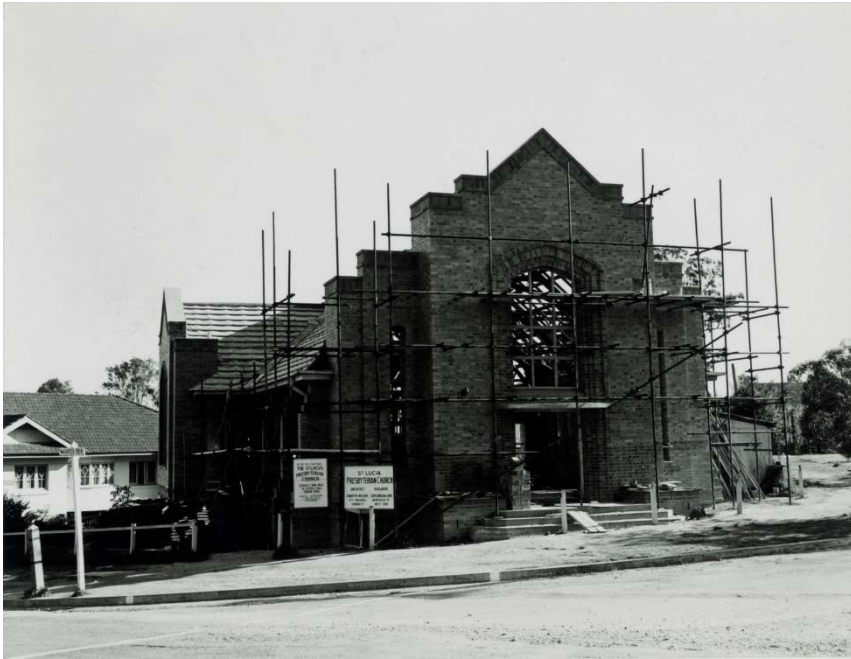
Left: Construction of the St Lucia Presbyterian Church [architect R.M. Wilson, built 1952], Queensland, n.d. Image no. 6523-0001-0341
